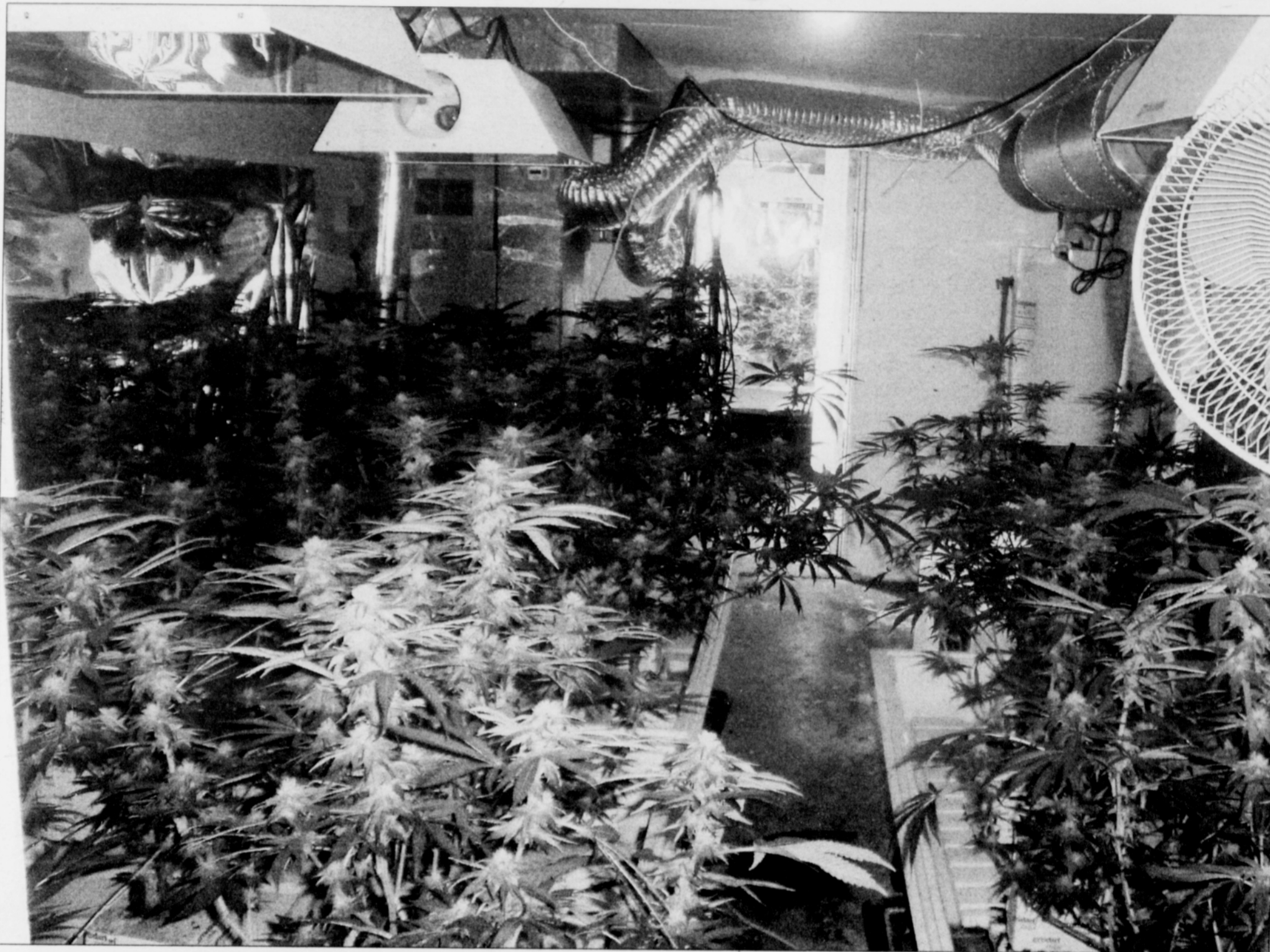
A Portland police photo shows a marijuana manufacture operation that was one of several grow houses specifically renovated for large-scale marijuana grows, many of which were not occupied by any residents.
