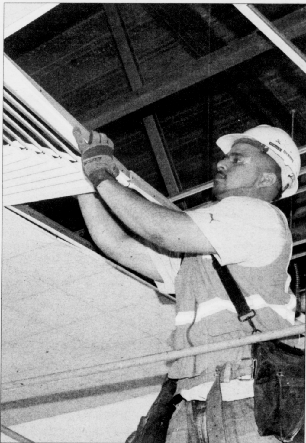
Ivan Ibanez of In Line Commercial Construction demolishes a ceiling during a remodel of the Student Service Building's third floor at Portland Community College's Cascade Campus.
