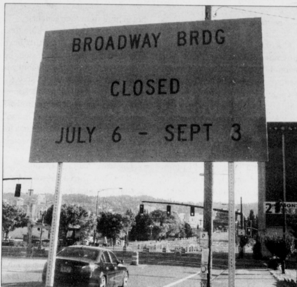
PHOTO BY DREW DAKESSIAN/THE PORTLAND OBSERVER Construction of the first modern streetcar line coming to the east side of the Willamette River along Broadway and across the Broadway Bridge closes the bridge to traffic through Sept. 3.
