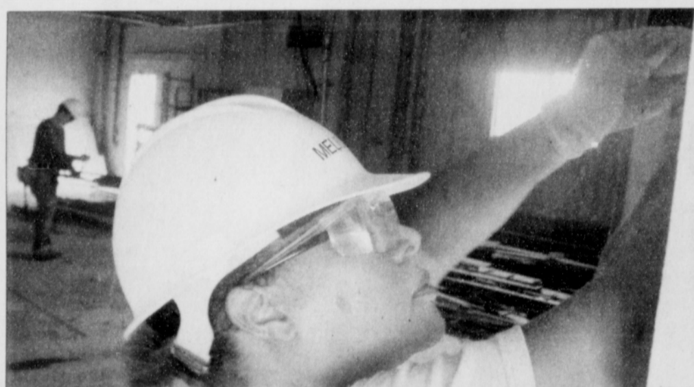
Melissa Jackson uses the claw of a hammer to tear down part of an old wall. Before enrolling in Oregon Tradeswomen, Inc. training program, Jackson worked in mortgage services. PHOTO BY JAKE THOMAS/ THE PORTLAND OBSERVER
