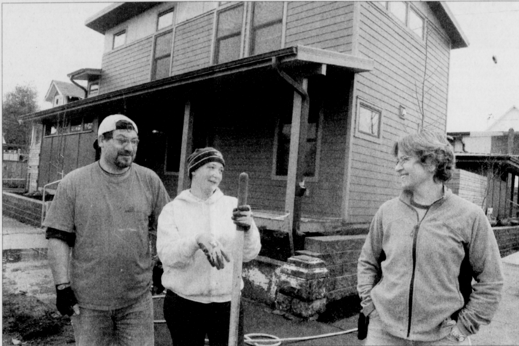
Juan Gonzalez (from left), Carrie Davis and Thea Zander work on a Habitat for Humanity home at 602 N.E. Webster St., the non-profit group's first LEED (Leadership in Energy and Environmental Design) home in Oregon.
