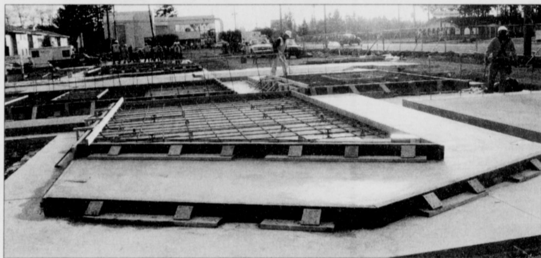
The foundation has been poured the walls are in the process of being poured for the new Salvation Army Gresham Corps Community Center.
