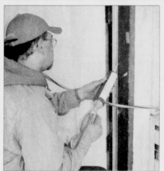
Cold air from a leaky door frame is sealed up with caulking.
