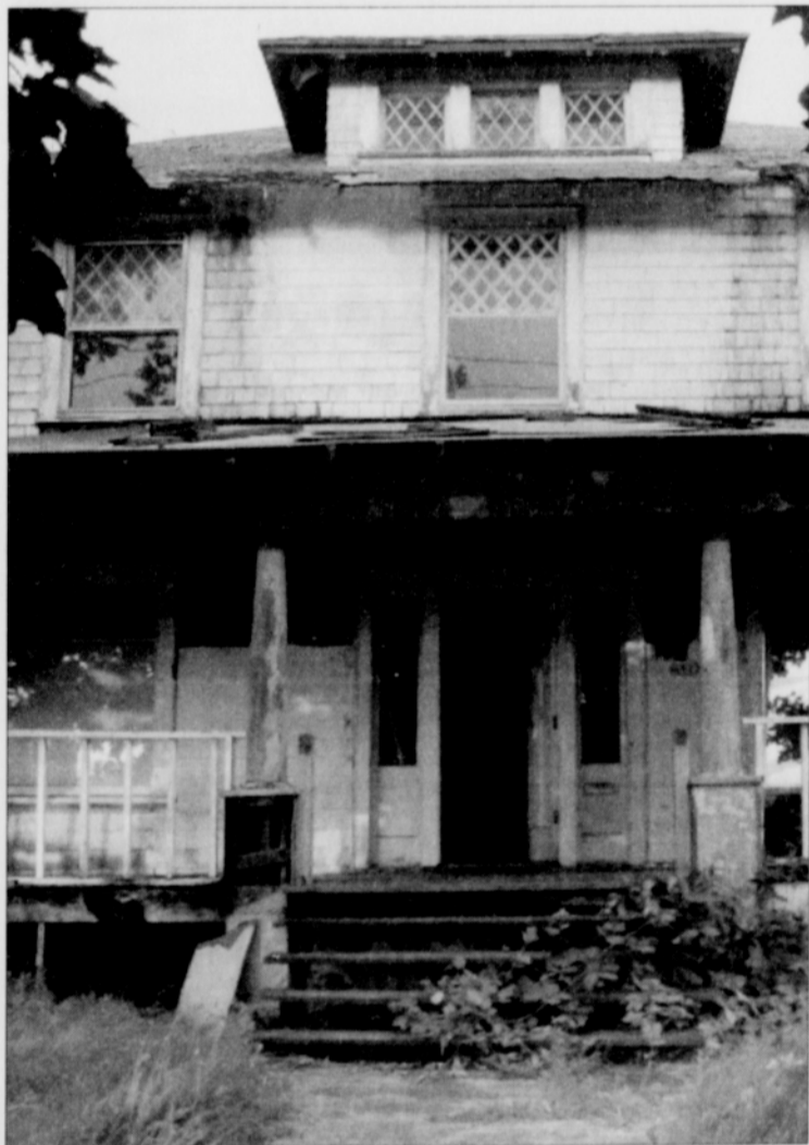
A house at 4922 N. Vancouver was in a serious state of disrepair when it was purchased two years ago for the future home of the North Portland Wellness Center.
