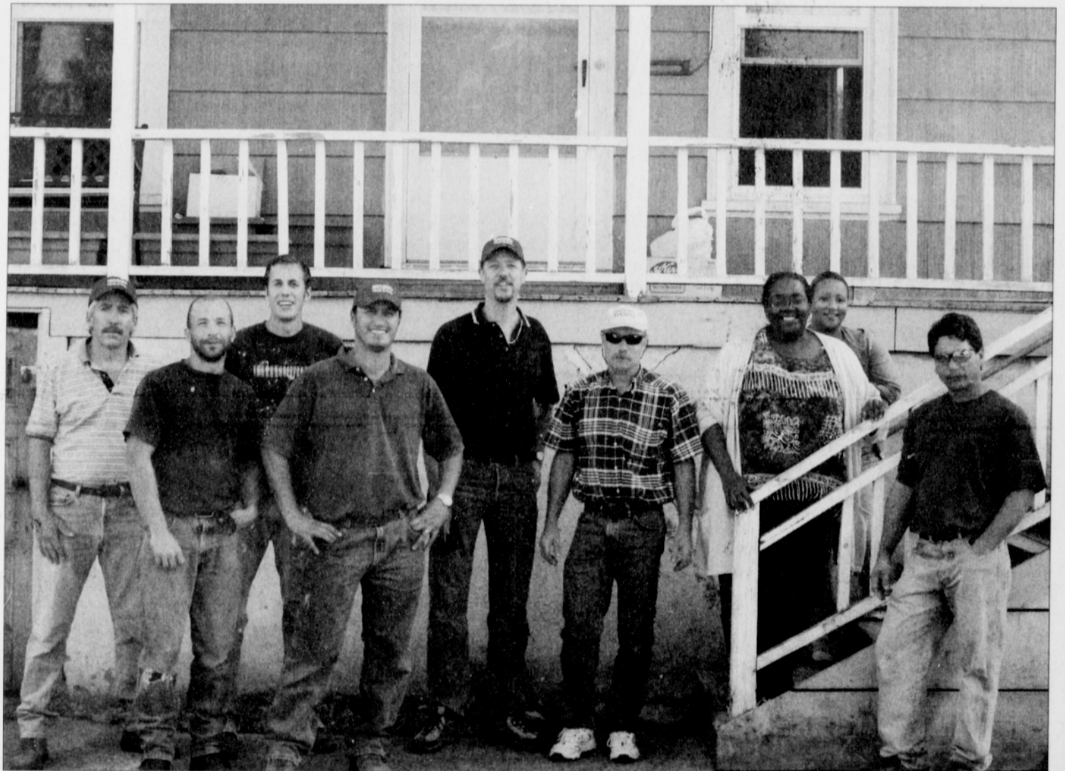
Doris Council (third from right) and her daughter Bryn (second from right) join Marty Smit (center) and the Affordable Home Remodeling crew after completing window installation in Council's home.
