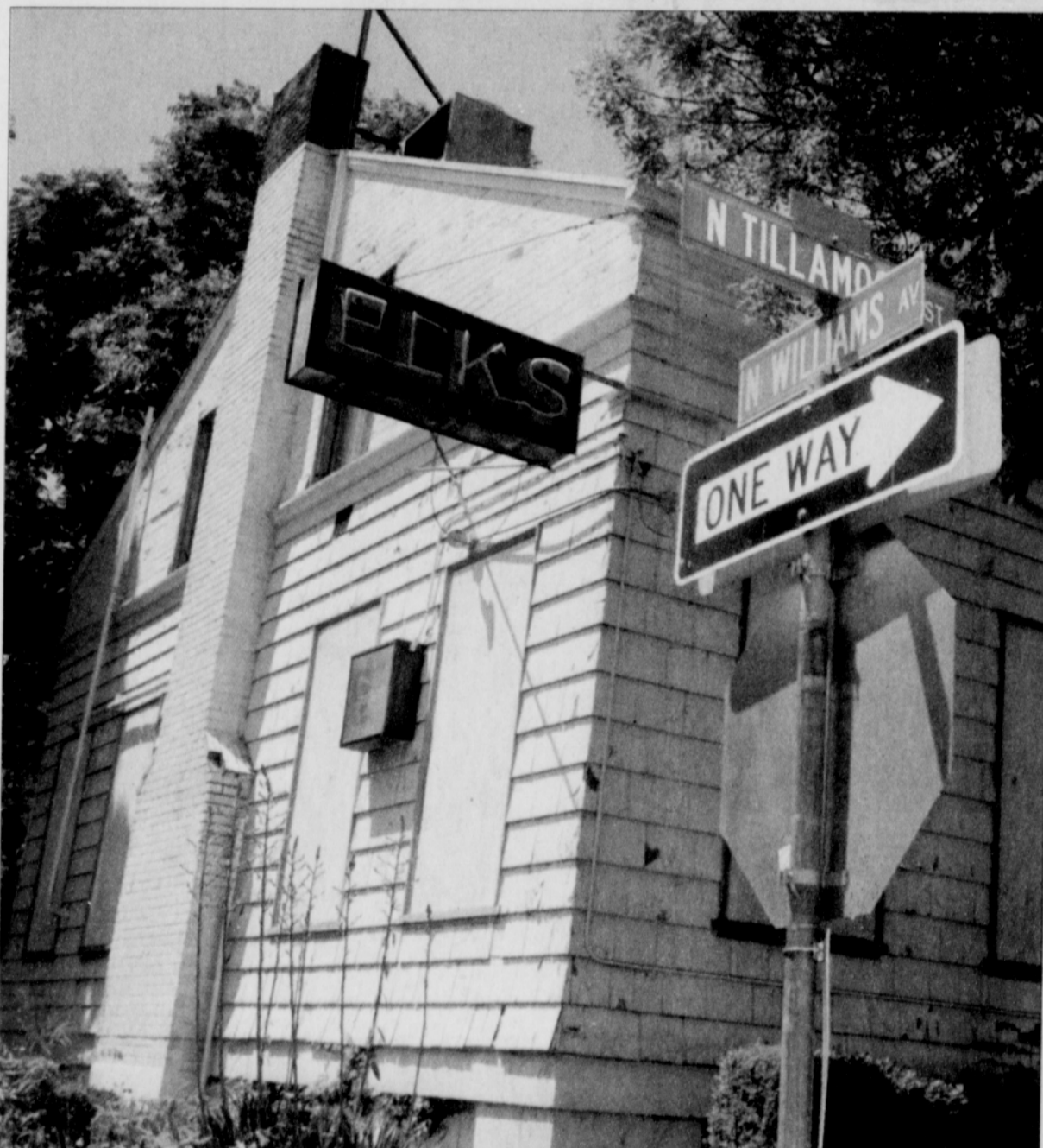
Restoration is coming for the historic and crumbling Billy Webb Elk's Lodge, a 1921 structure that once served as a YWCA for black residents.
