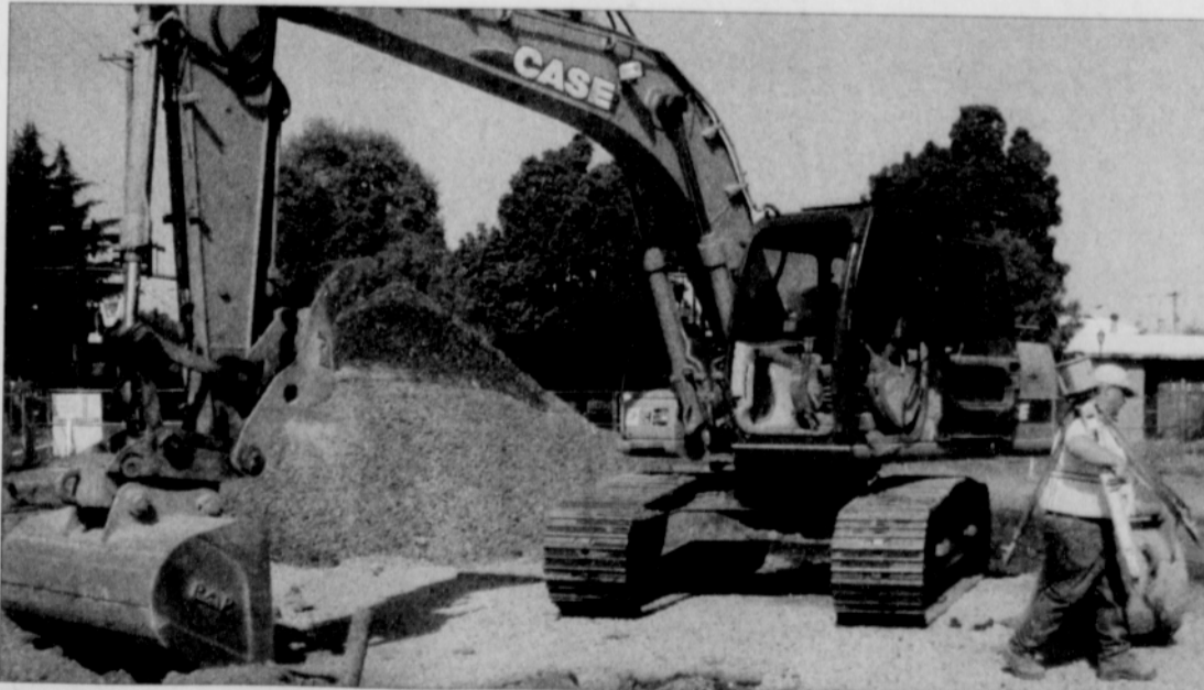
PHOTO BY MARK WASHINGTON/THE PORTLAND OBSERVER Groundbreaking has begun for a new mixed-use storefront at Northeast Fremont and Martin Luther King Jr. Boulevard, bringing economic vitality to long blighted block.
