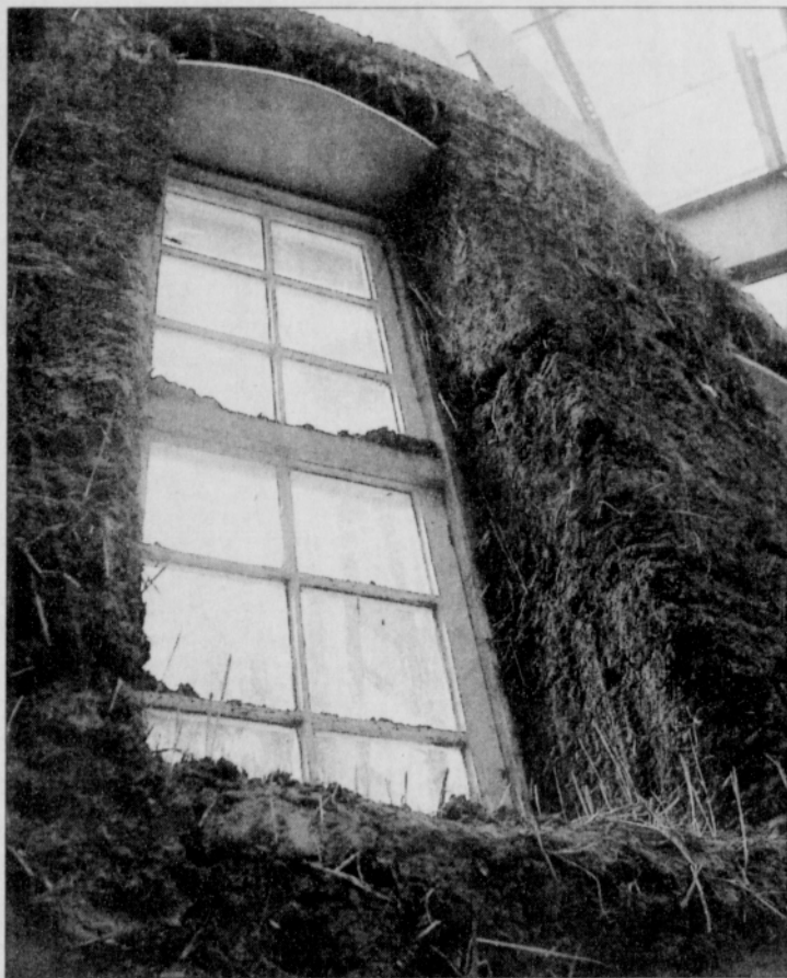
A wall made of straw and mud is under construction at the ReBuilding Center on North Mississippi. The wall is complete with reused windows and shelves and serves as an entrance into the public center.
