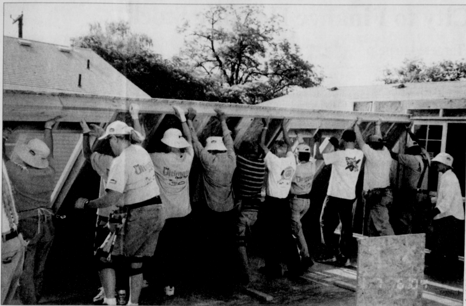
All hands are needed when the walls go up on a local Women Build project that adds much-needed affordable housing to the community.
