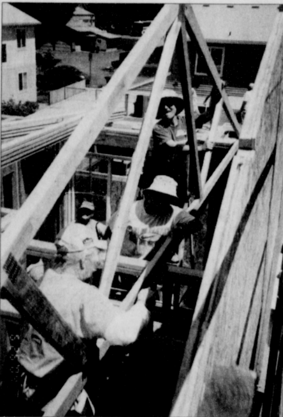
Women of all ages and abilities feel empowered during the construction of a home.
