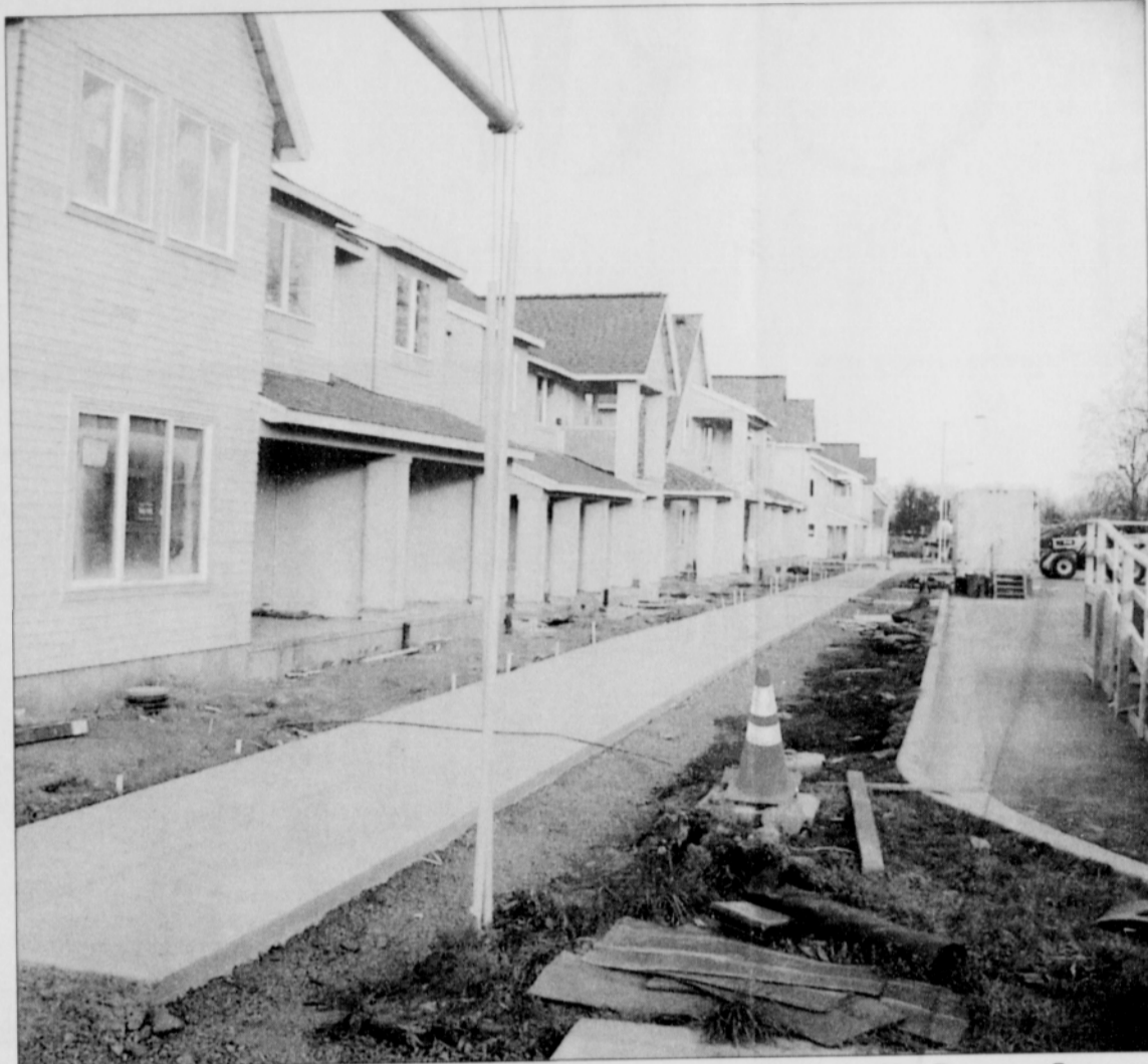
PHOTO BY MARK WASHINGTON/THE PORTLAND OBSERVER New streets and sidewalks better connect New Columbia to the surrounding Portsmouth neighborhood of north Portland.
