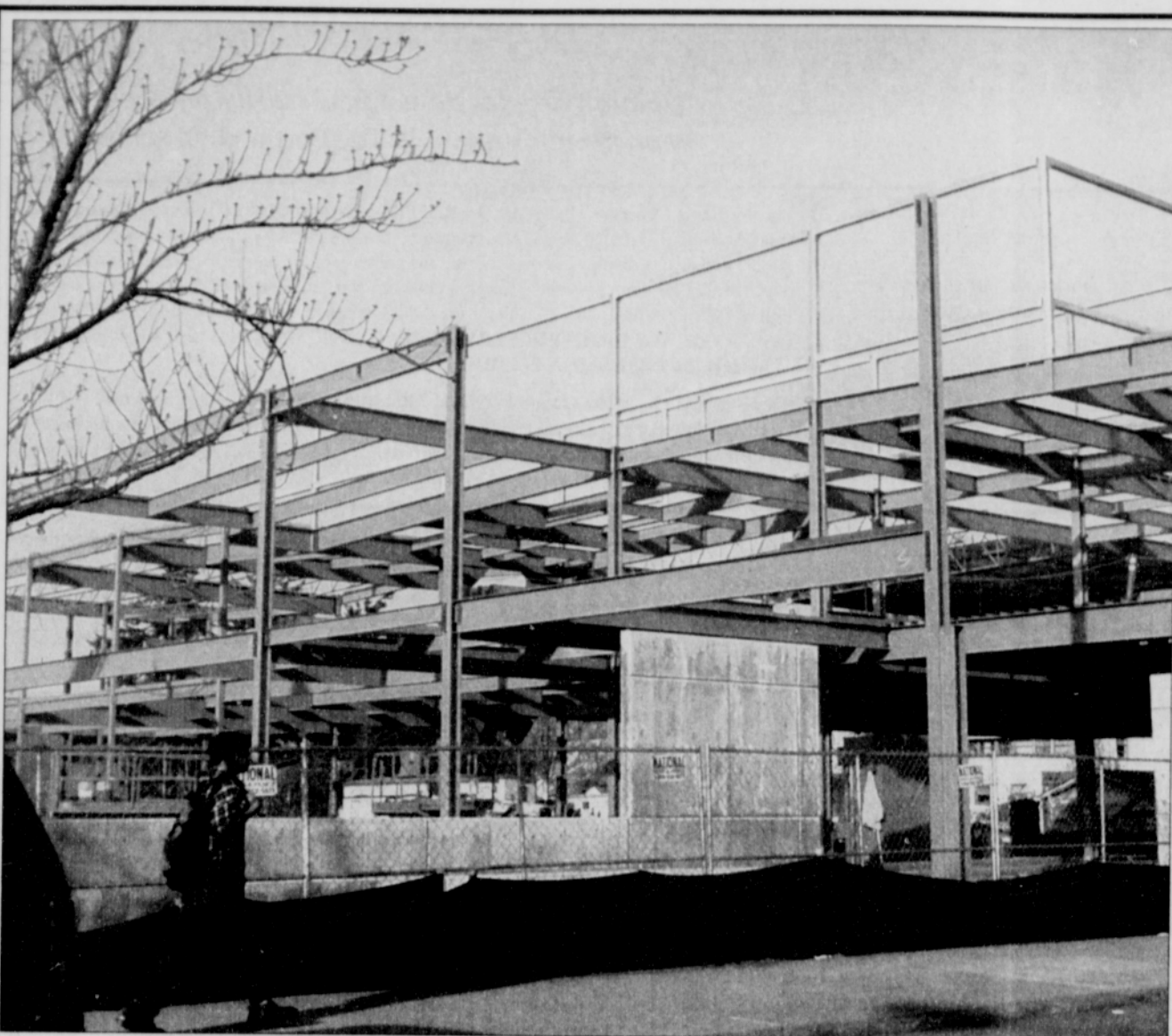
A student walks past the construction of a new Technical Education Building in the center of the PCC Cascade campus that borders North Killingsworth Street. The construction is part of $57 million in campus project. Eventually five new buildings on the campus will expand student services, increase access to adult learning programs and add instruction in workforce development skills.
