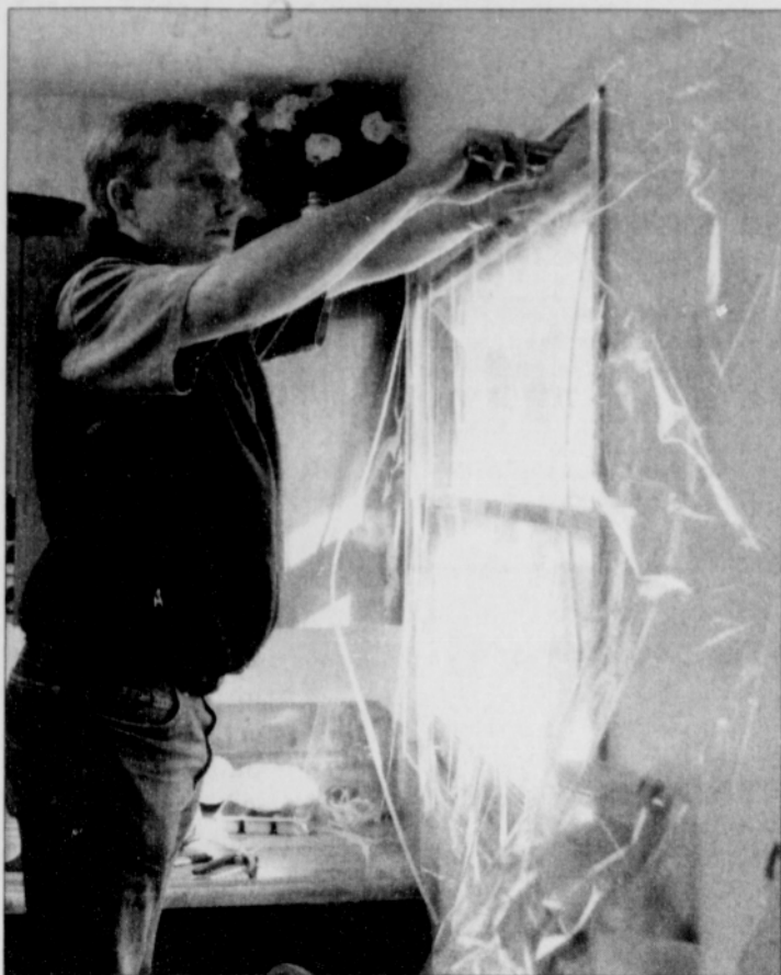
Portland General Electric Employee Rick Weijo installs vinyl storm windows on the north Portland home of Elmer Miller.
