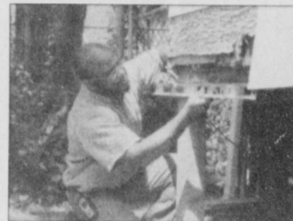
Vernell West of VWESTCO checks the level of a back porch that has begun leaning over time, a common problem in many older homes where porches were converted to living quarters.
