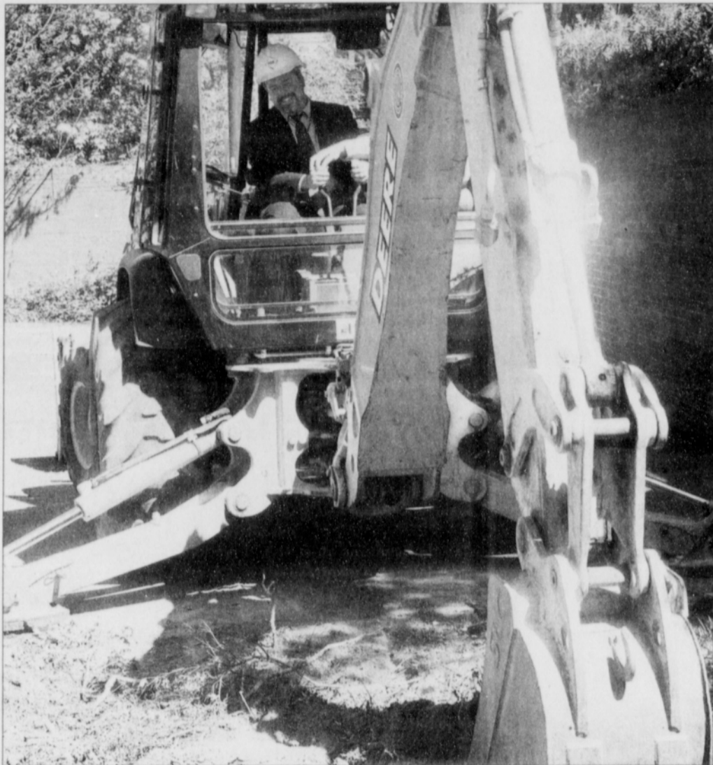
Oregon Burn Center Medical Director Dr. Nathan Kemalyan begins the excavation process for the Therapeutic Garden aboard a PGE blackhoe.
