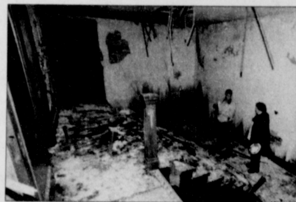
The dilapidated interior of the former Masonic Lodge across from Jefferson High School in north Portland. The non-profit music group Ethos, Inc. won a bid to purchase the building from the Portland School District. It plans a complete renovation of the historic structure.
