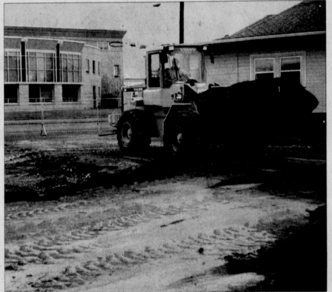
Workers for minority contractor Alexander Adebawo level land where the Cascade Campus of Portland Community College has expanded on the south side of North Killingsworth to accommodate a new athletic center. PHOTO BY MARK WASHINGTON/THE PORTLAND OBSERVER
