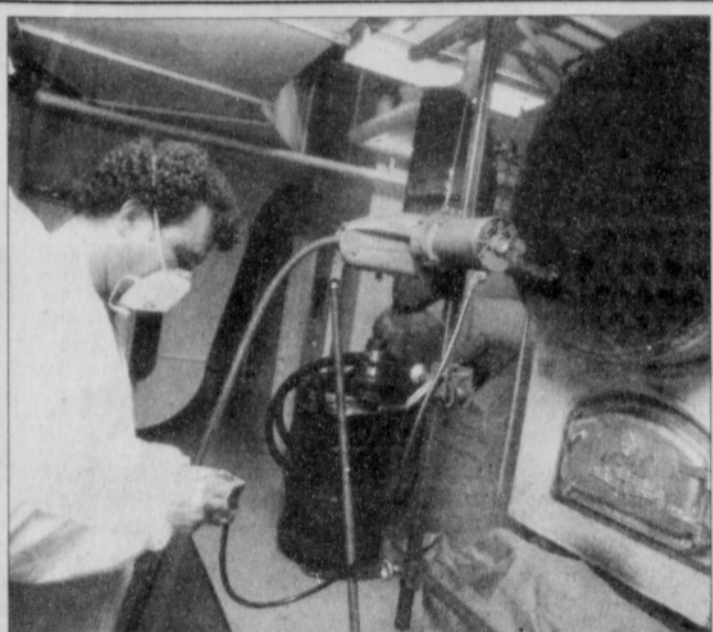
Astor Middle School custodian Dan Strong wears protective clothing as he prepares to "punch" a boiler. The cleaning process that keeps soot out of the ventilation system is vital to students' health.
