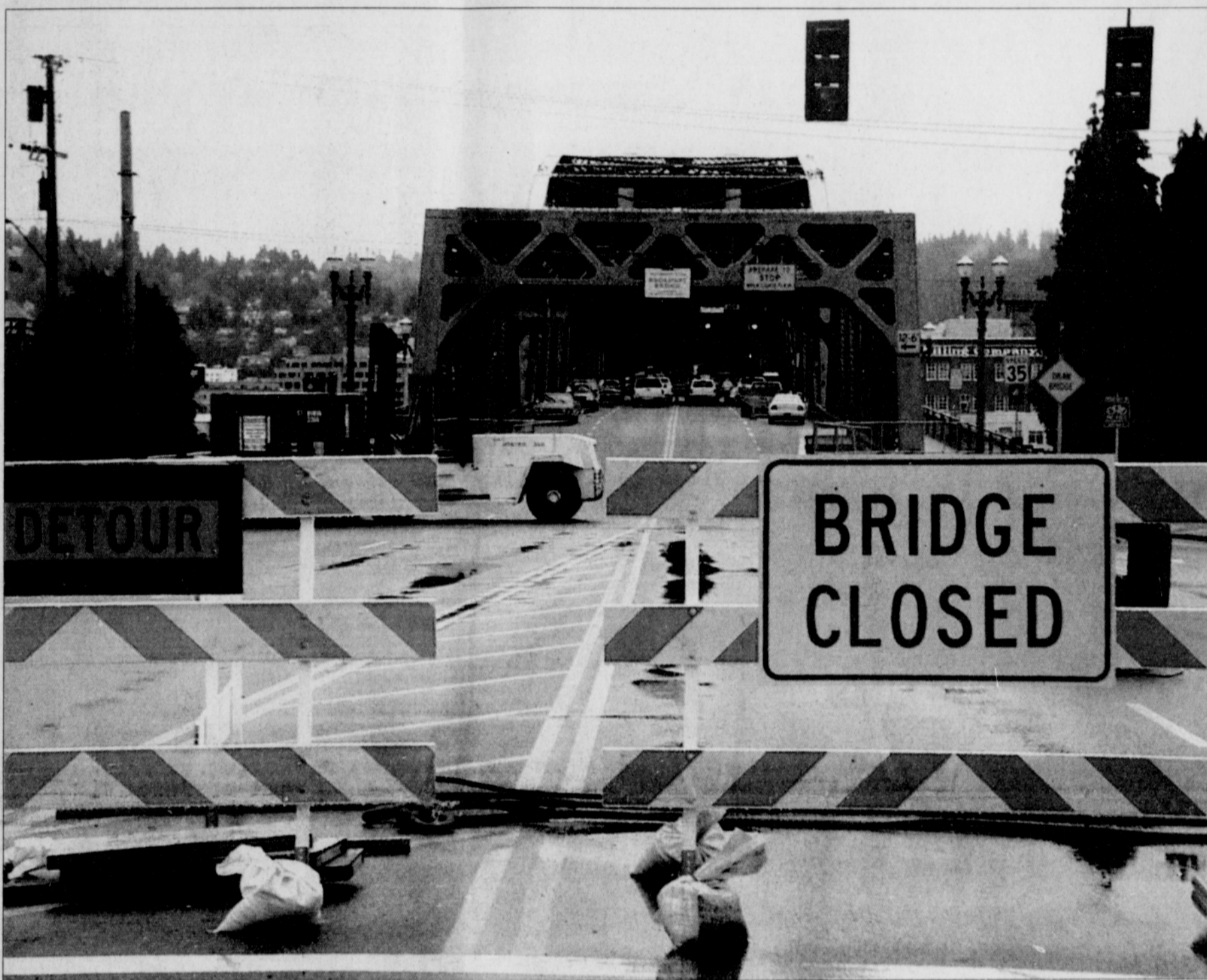
Currently, the Broadway Bridge is completely closed due to repair work. It will reopen before the end of the month. A construction crew is busily replacing the original mechanical parts that allow the bridge to open and close for ships. The original parts were installed in 1912. Much more extensive work will be done to the Broadway Bridge in April of 2003, that would last twenty-one months. Total closure for the project would be for two months. The upcoming project calls for repainting part of the bridge, repairing the deck where cars pass through, rebuilding the sidewalks and replacing the steel grating with a solid grating in the center of the bridge.
