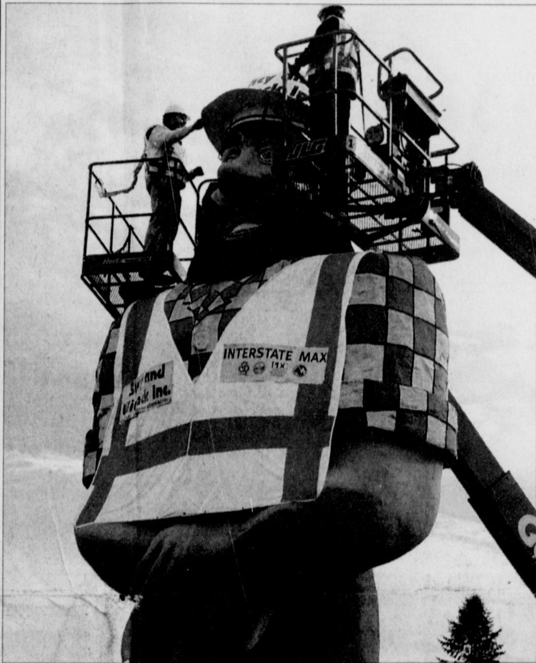
Paul Bunyan is fitted with a construction vest and hat in preparation for a big move in the Kenton neighborhood of north Portland. The 43-year-old statue will be moved 50 feet on Monday morning at 8:30 a.m. to make room for the Interstate Max Light rail project. Jerry Buxbaum of Studio 23 Productions made Paul's safety gear. The company specializes in visual concepts for print, video and special events.
