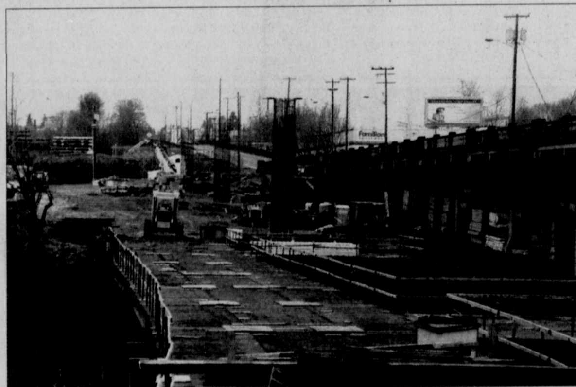
A new bridge under construction in north Portland will carry MAX light rail trains over the Columbia Slough near Denver Avenue.
