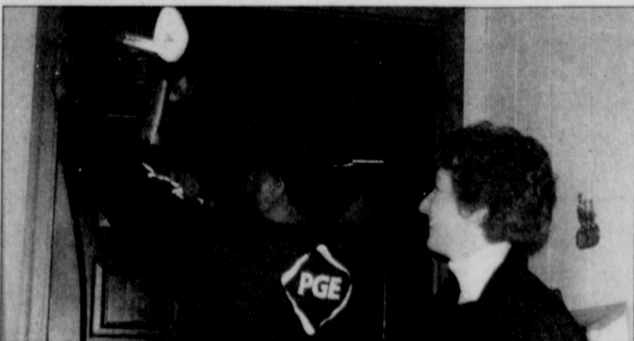
A volunteer from Portland General Electric fastens weather stripping to the door of a southeast Portland home as part of a campaign to help senior and disabled residents lower their energy costs.
