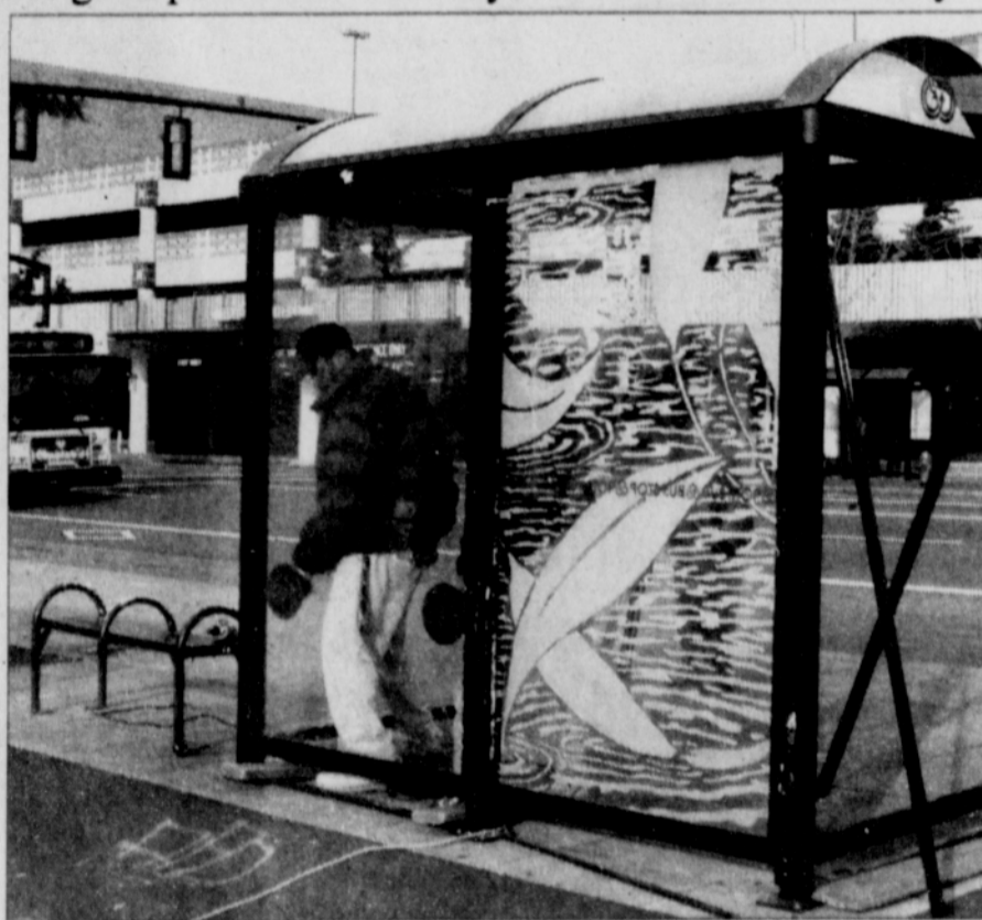
Jordan Greene of Warren Pacific Corp. removes a graffiti-damaged glass panel from a Tri-Met bus shelter near Lloyd Center Cinemas. It will be replaced with an artistic panel like the one on the right.
