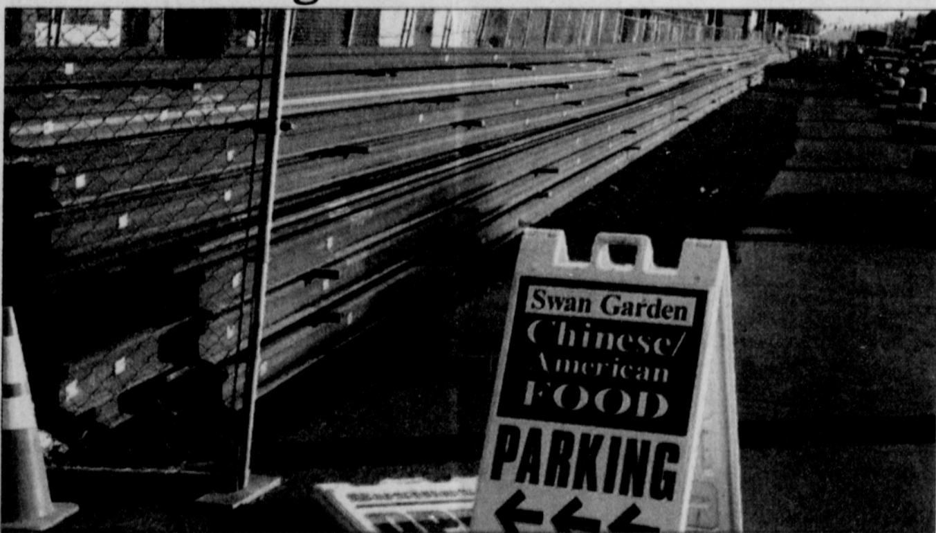
Businesses along Interstate Avenue in north Portland use signboards to guide customers around stockpiled rail and other obstacles during the construction of a 5.8-mile long light rail line from the Rose Quarter to the Expo Center. TriMet hopes to alleviate some of the confusion with a new "Open for Business" campaign.
