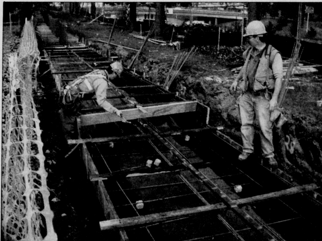
Crews prepare the footings for soundwalls just north of Skidmore as part of the Oregon Department of Transportation's I-5 Preservation Project. Crews are also relocating utility lines, forcing some closures in the streets adjacent to the freeway. Restricted traffic is also in effect on the Lombard and Portland Boulevard overpasses as crews work to raise the structures to allow better clearance for freeway truck traffic.
