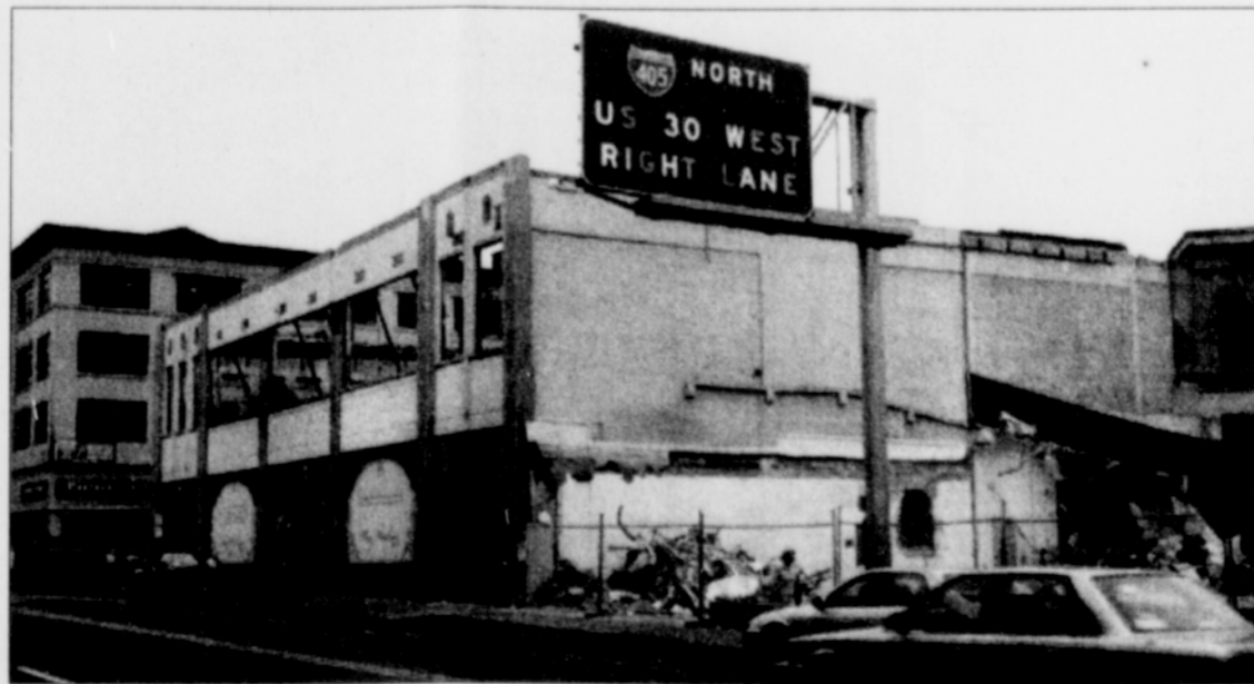
The administrative office building the day before demolition was scheduled to occur.
