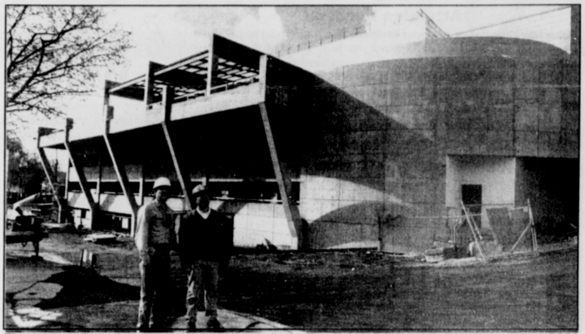
The outer walls and roof are now up on a medical office Kaiser Permanente is building in the 3600 block of North Interstate Avenue in north Portland. Observing the construction work are Hoffman Construction's Kelly Rowland, field superintendent, and Ken Pasley, project superintendent. Kaiser Permanente expects sometime this fall to open the two-story medical building, which has three stories of underground parking. Remodeling work on a 20-year-old medical office next door is slated for completion early next year. Photo by Carole Archer.
