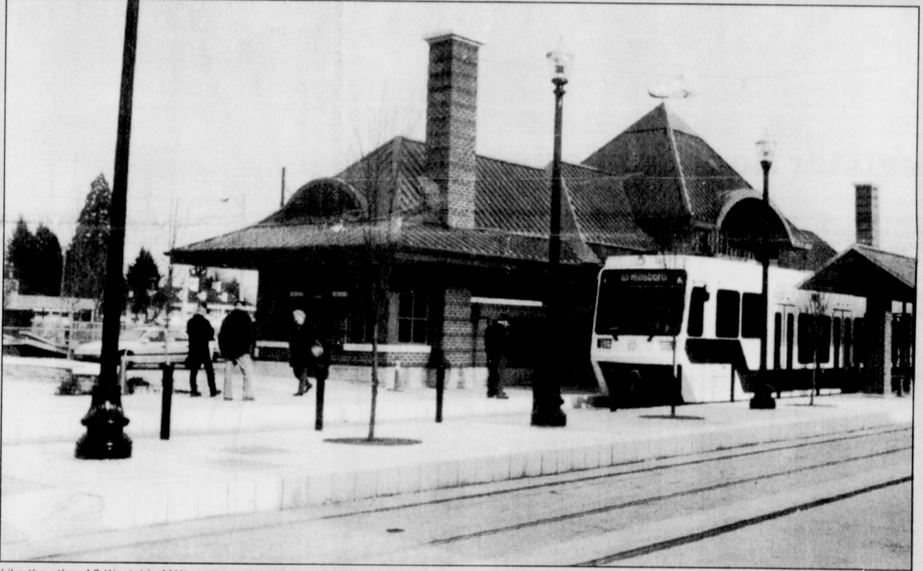
Like the other 19 Westside MAX stations, the Hillsboro Central Station building - on Washington Street near Third Avenue - is substantially complete. Electrical crews are hard at work in Washington County, stringing the overhead wire that powers the light rail trains, and installing signals and communication systems. They are scheduled to complete this work in April. At the same time, other crews are doing similar work in the three-mile, twin-tube tunnel under Portland's West Hills. The Grand Opening of the 18-mile-long Westside MAX extension is Sept. 12 and 13, 1998. (Photo by Mark Going).
