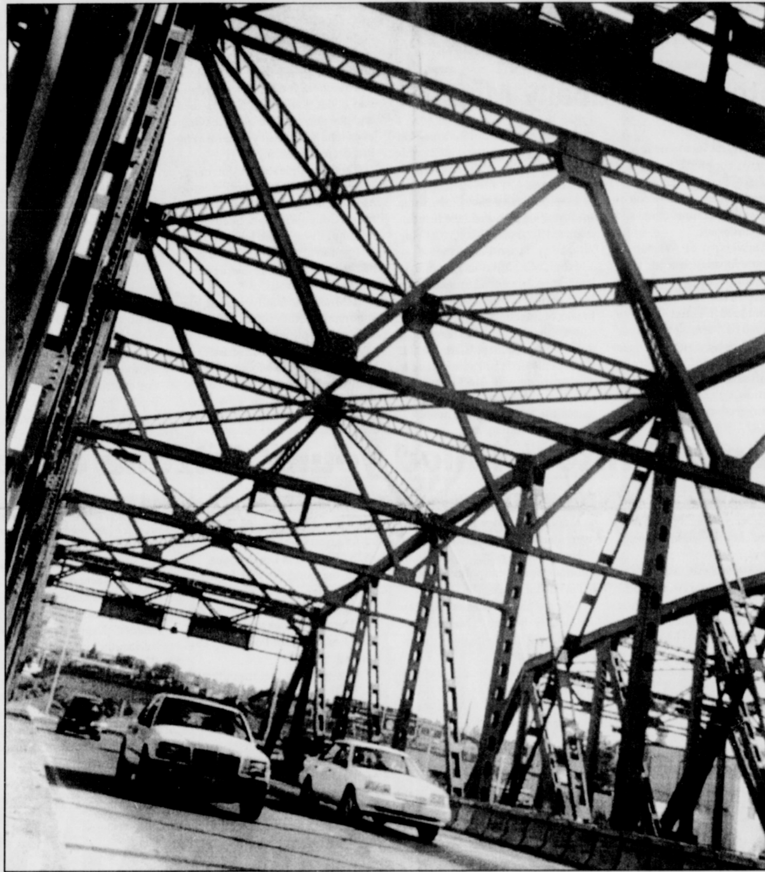
Portland and Vancouver traffic conditions during the repair of the Interstate 5 bridge may be worse than originally anticipated. This, according to Oregon Department of Transportation officials may occur as a result of last week's announcement to shorten the bridge closure time from 21 days to one week, giving commuters a sense they don't need to adopt alternate routes.
