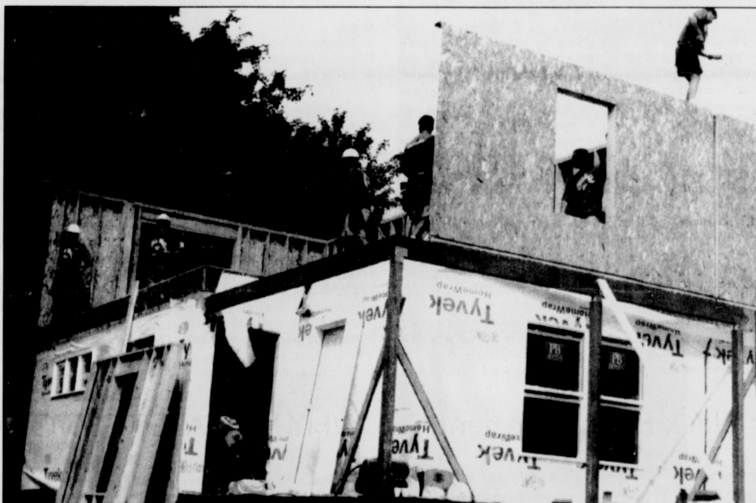
A team of professional builders set a record as they construct a two-story townhouse on Northeast Cleveland Avenue in just one day.
