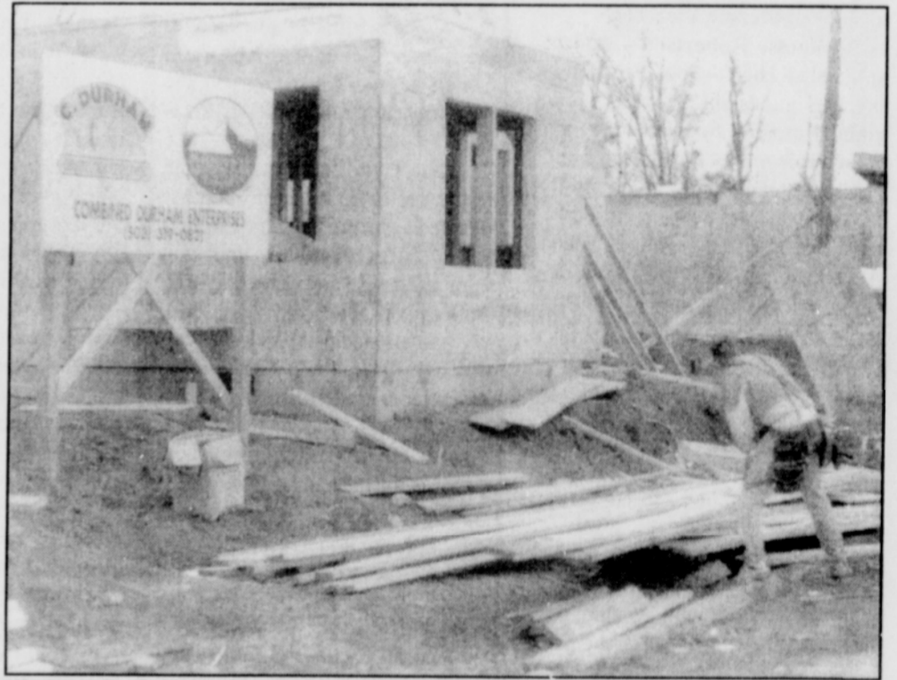
Workers for Durham Construction are building new homes in the King neighborhood on Northeast Roselawn.
