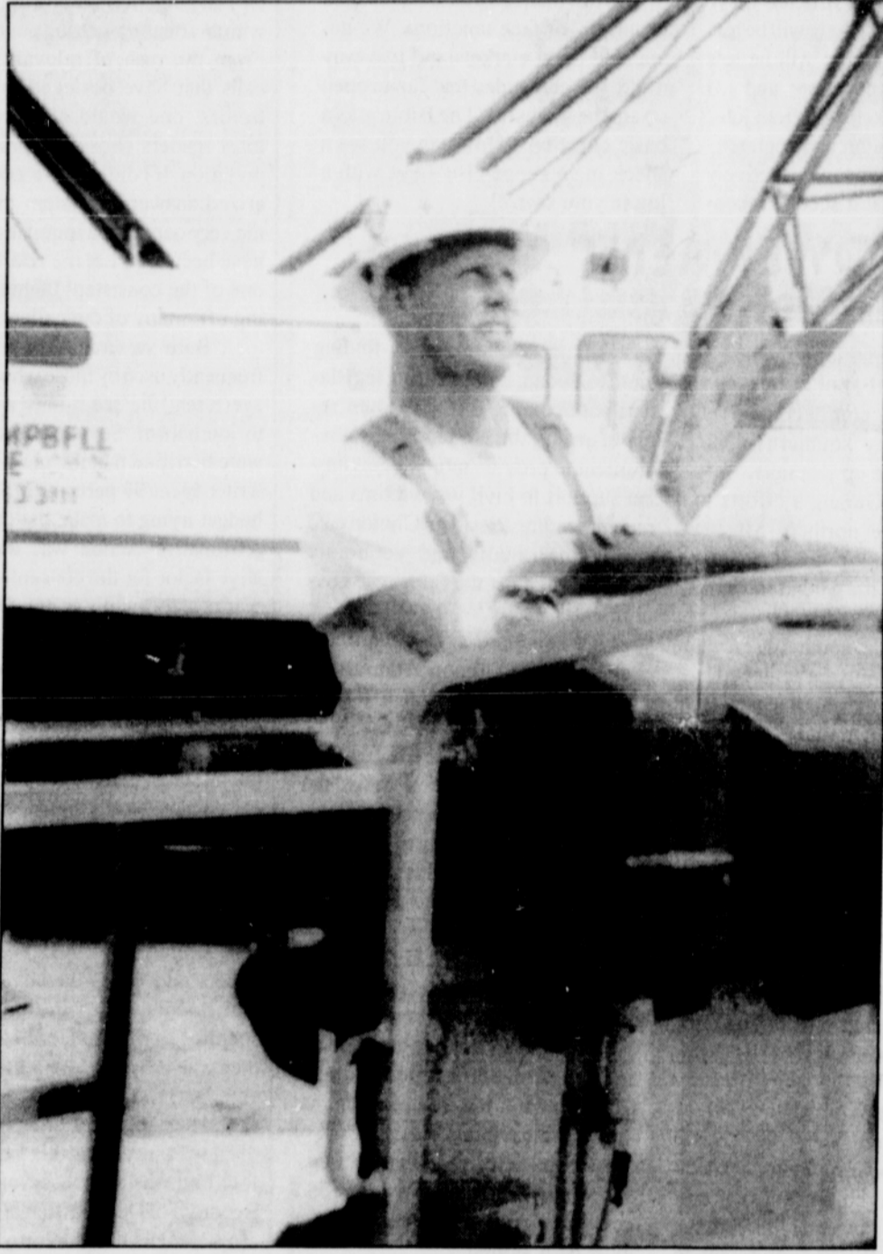
Tom Le Pley is part of the construction crew that will make the Blazer Boys and Girls Club a reality. Our roving camera was at the project site on Martin Luther King Jr. Blvd. this week. The $2.2 million, 27,000 square foot club will include a gymnasium, education wing and teen center. Support for the club came from the Portland Trail Blazers, other corporations and individual donors.
