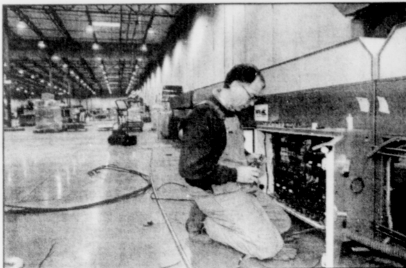
Installing wiring for production equipment at Portland's new Rundel Products manufacturing and warehouse facility is Jim Reed, a member of the International Brotherhood of Electrical Workers, Local 48.
