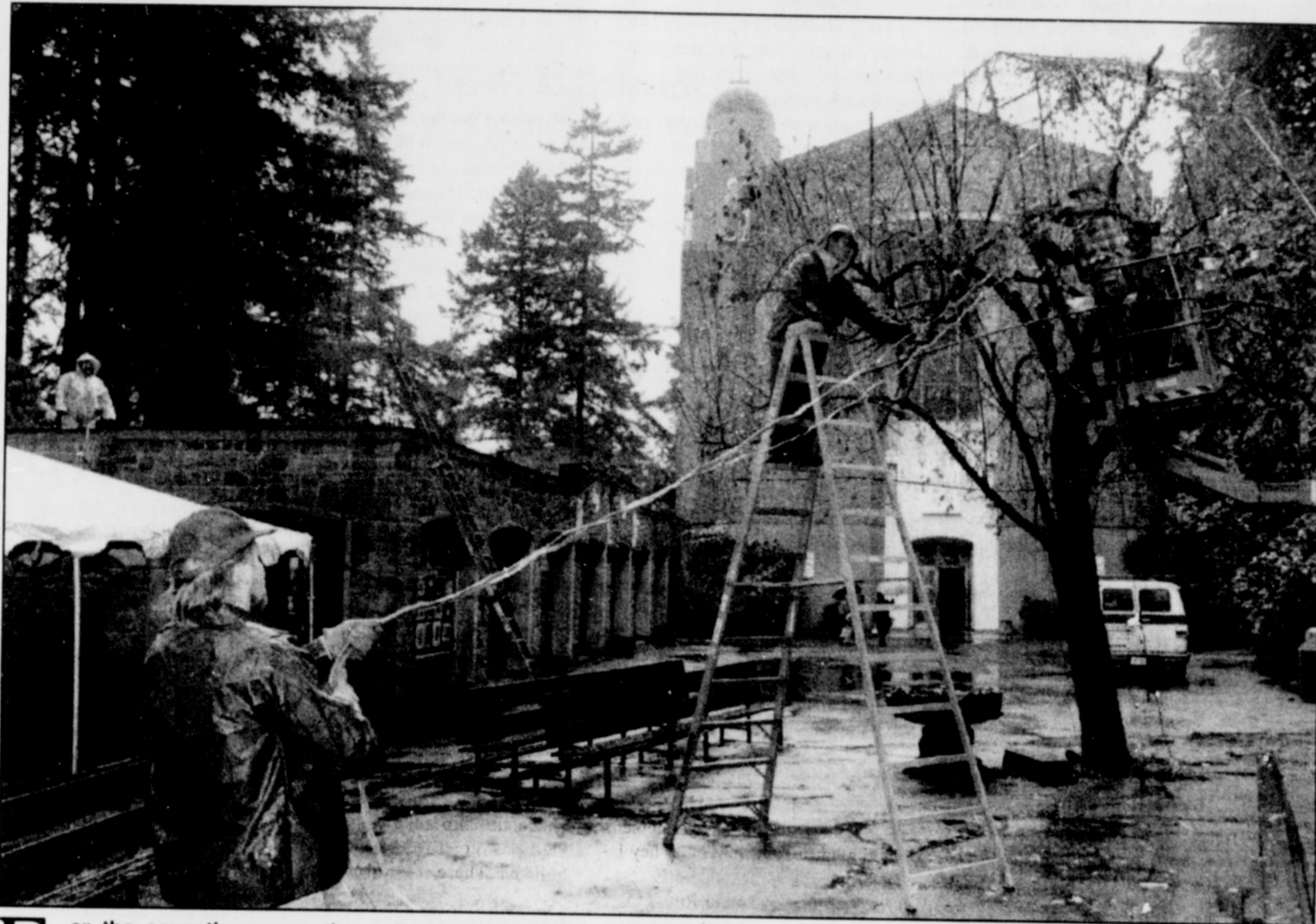
Volunteers from the National Electrical Contractors Association (NECA) and the International Brotherhood of Electrical Workers (IBEW) Local 48 donated labor and materials to light The Grotto for the sanctuary's annual 'Festival of Lights' Christmas celebration. The 27-person volunteer crew included IBEW Local 48 Electricians from Sunset Electric, Cherry City/Morrow Electric, Electrical Construction Company, Chandler Electric, Far West Electric, Christenson Electric, Tice Electric, and Atlas Electric, all members of NECA.
