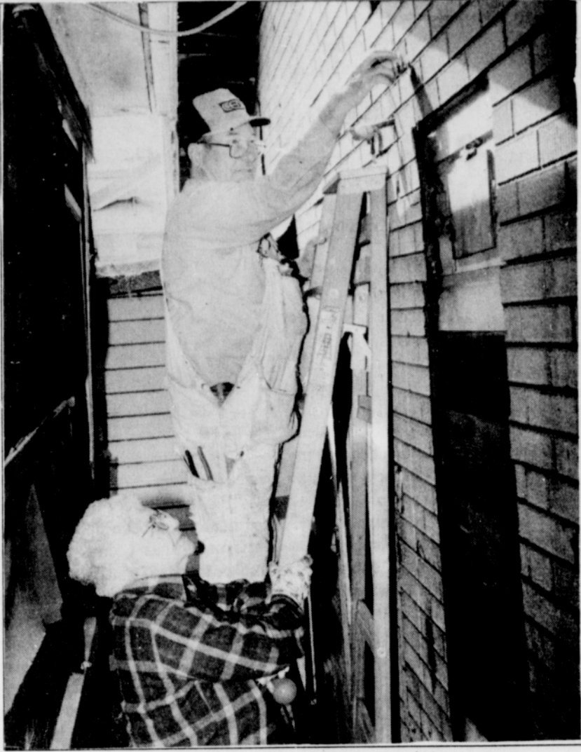
Chuck Burns, volunteer coordinator for the Christmas in April electricians and a retired IBEW member, replaces unsafe wiring while homeowner Harriet Clausen inspects his work.
