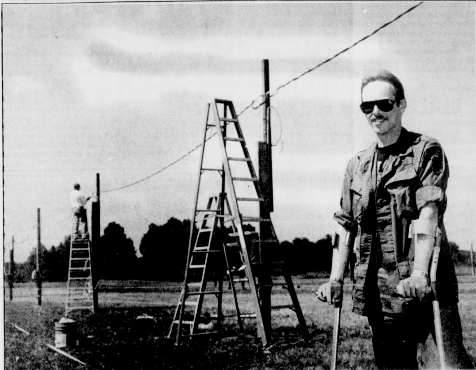
Mark McMurtrey, employment specialist with the Disabled Veterans Outreach Program, looks on as IBEW Local 48 electrician Jake Harding installs wiring for Portland Stand Down 1993, an event that provides services for homeless vets.
