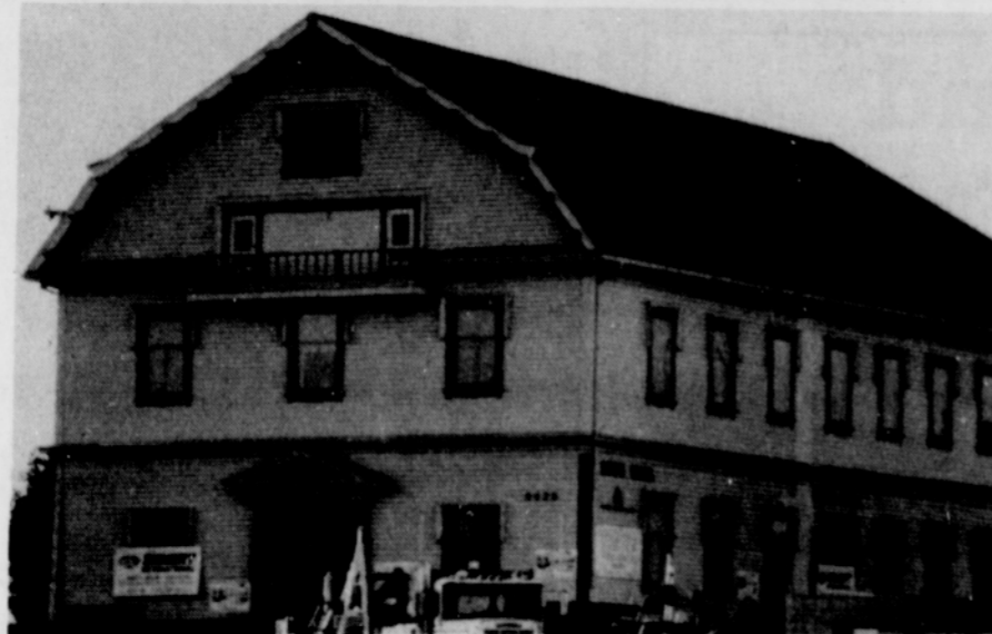
The 83-year-old Town Hall in north Portland begins moving to its new home on the Edgar F. Kaiser Health Center. Built by Finnish immigrants, the education and conference center was moved by Kaiser Permanente
