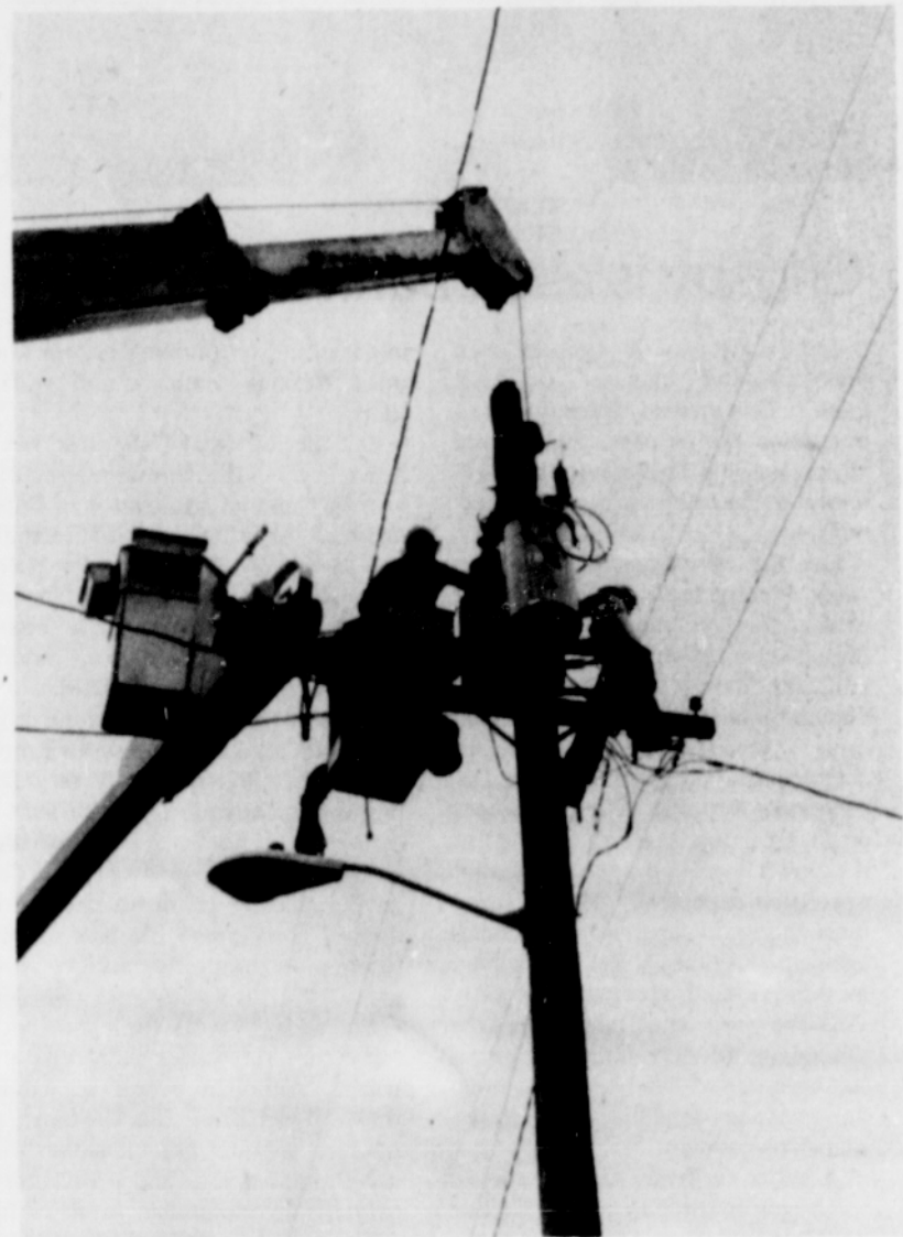
Removing old transformer after installing a new one. PP&L journeyman linemen in "bucket" and on pole work high above street level. Linemen are skilled in safety measures as well as electrical procedures.
