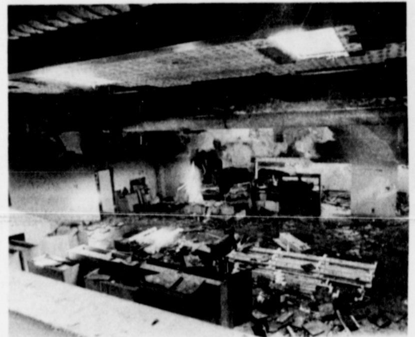
The new wing of Tubman Middle School suffered severe damage in Sunday's arson-set fire. (Photo: Richard J. Brown)
