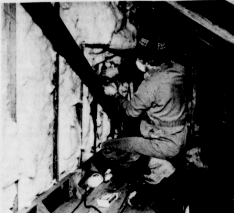
Installing insulation in the James Canyon residence; part of Overlook neighborhood's weatherization drive.
