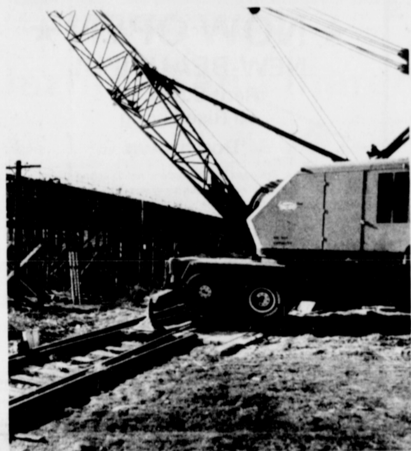
Hatch heavy equipment readies for Banfield project work. (Photo: Richard J. Brown)
