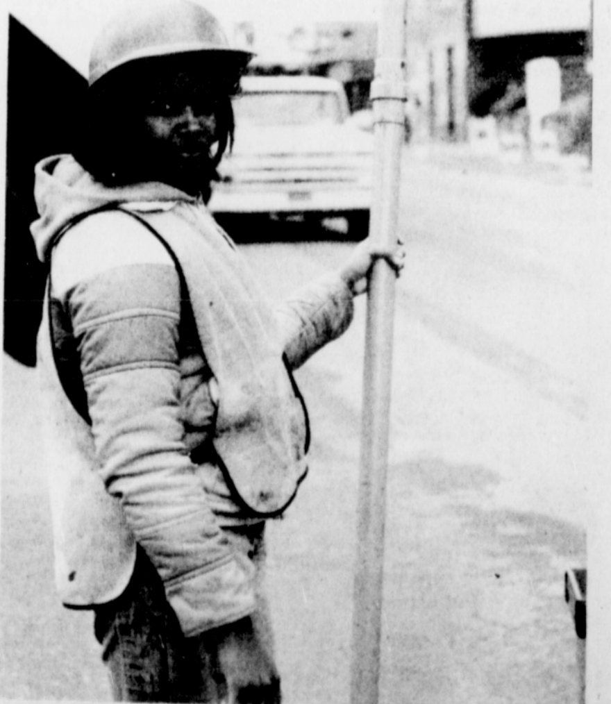
Flagwoman Bonnie Thomas helps control the flow of traffic thru the Union Avenue construction site.
