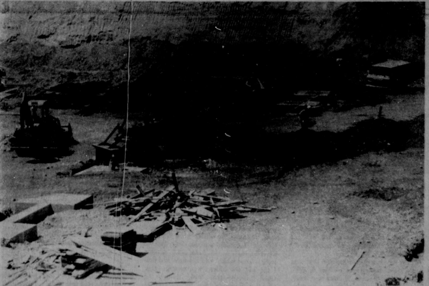
Construction crews are busy at Portland Public Schools' Educational Center construction site.
