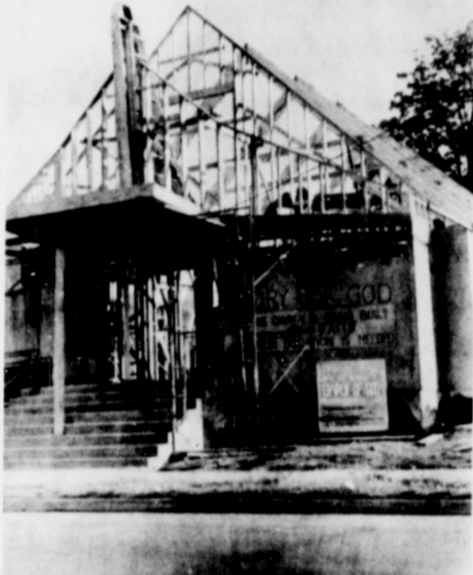
The Ark of Safety Church of God, Inc., is building at N. Killingsworth Avenue. The church, pastored by Bishop U. B. Peterson, is being built by the members of the congregation. Services are already being held in the home of the new structure.
