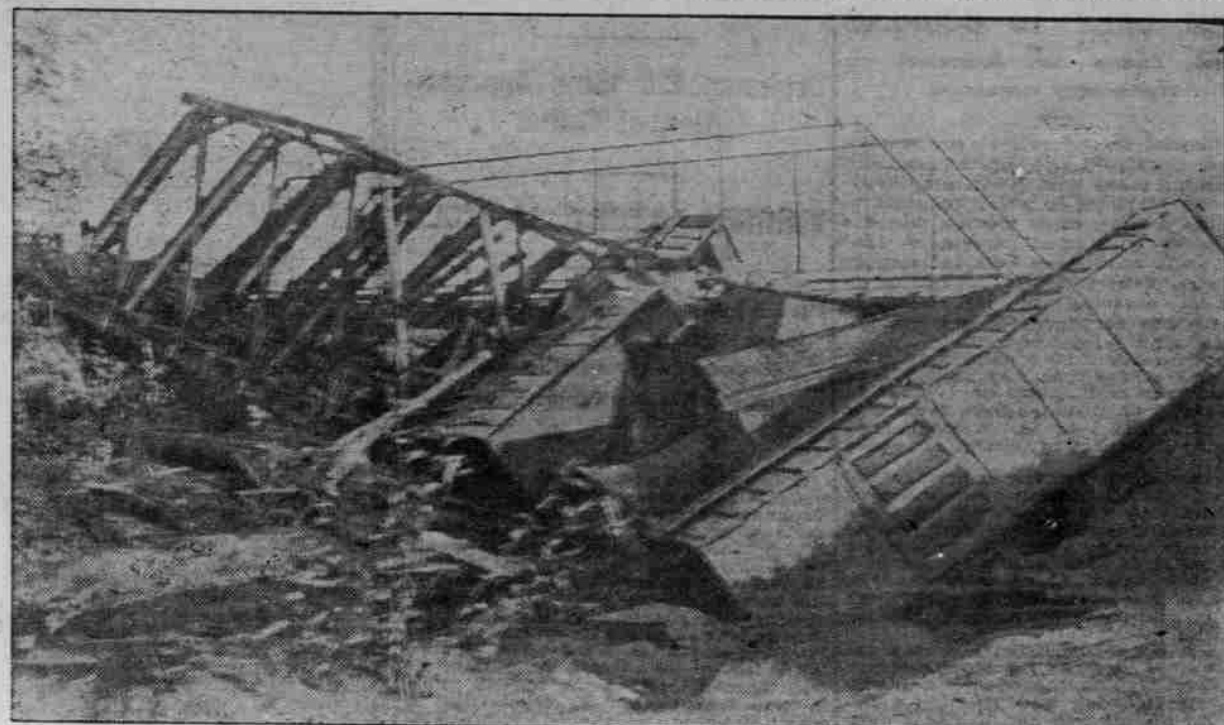
BROKEN BRIDGE WITH CARS LYING IN CREEK. ELMA, Wash., Oct. 31.—(Special).—Early Saturday morning the "highball" freight on the Milwaukee, going west, was wrecked when the bridge across Delezeze Creek gave way. Twelve cars went through the bridge and piled in a heap in the creek. All were empty except one, loaded with general merchandise. The damage was probably caused by one car being off the track, having run that way for a considerable distance until it struck the bridge and toppled over, causing the wreck. No one was hurt. The wrecking crew from Tacoma were at work three hours after the accident.
