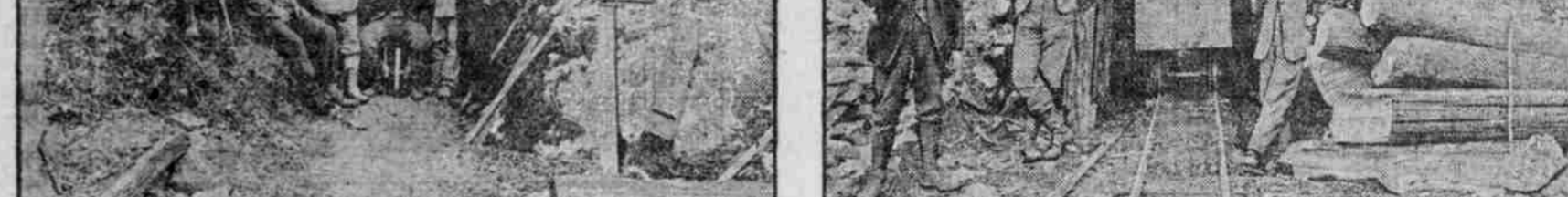
Entrance to Tunnel No. 3, in 500 feet, showing car track and dump cars.
