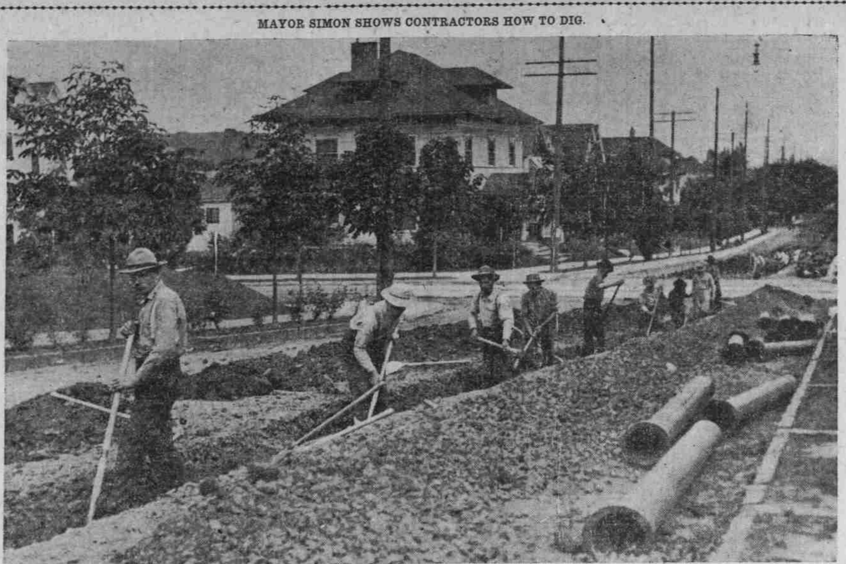
MEN AT WORK ON WATER MAIN ON EVERETT STREET UNDERTAKEN BY CITY HEAD HIMSELF. As a contractor, Mayor Simon is teaching competitors how to lay a water main quickly. As will be seen in the accompanying photograph, he has a large force of men at work in Everett street installing an eight-inch main from Twentieth street to Cornell road. This is the job the Mayor tackled when certain contractors bid exorbitantly, the Water Board having authorized him to submit a proposal if he deemed it wise that was due to him. As we all know, his was a short life and taking into consideration all that he accomplished, more notice should have been taken of his great deeds.
